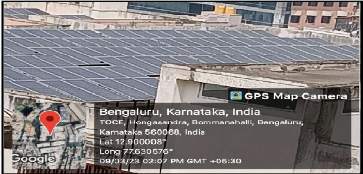
Overview of Solar Panel
